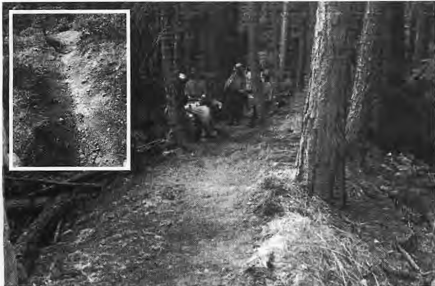
Trail crew at work on the Pioneer Trail in Northern California, site of the Wild West Ride. Inset: the old, deteriorated trail.
